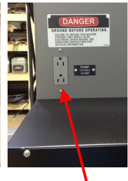
120VAC receptacle for pump
